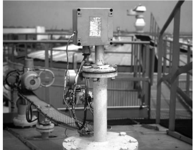
Fig. 12b. Example of a Temperature Measurement Instrument (HIMS installation)
